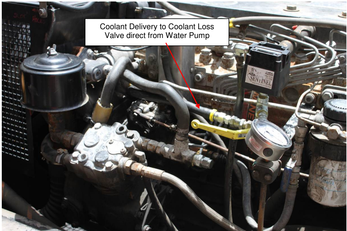
Figure 2: Alternate Coolant Loss Valve Setup – Brumby Installation (with gauge installed for testing).
