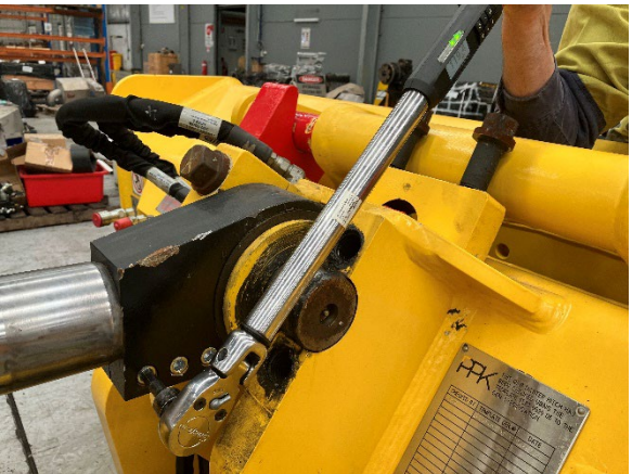
Figure 9. Repeat the replacement sequence for bolts 2 & 3 then check bolt torque of 120 Nm in same sequence.
