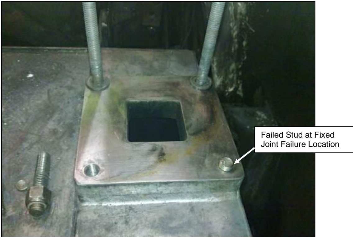
Figure 3: Photograph showing the failed stud at the fixed joint failure location between the purifier and the scrubber.
