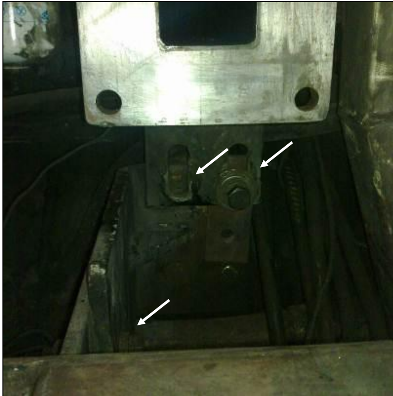
Figure 5: Photograph highlighting the apparent movement of the fastened supporting bracket assemblies.
